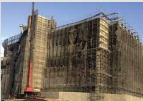
Tung Ho Steel Plant, Taiwan
