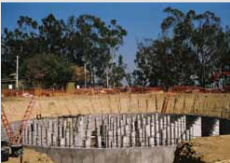
TreePeople Center Cistern, USA
